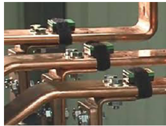
Figure 1.8. Set of Easergy TH110 sensors fixed on the 3 phases of an electrical connection
